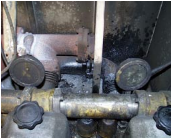
FIGURE 6 Residue of fuel oil spray within exhaust casing
