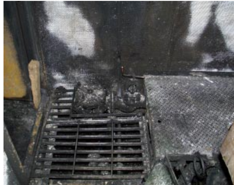
FIGURE 3 View of port side of generator space – looking aft to steering flat
