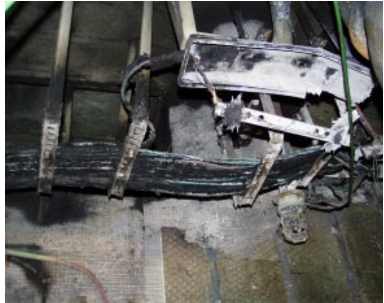
FIGURE 5 Fire damage to deckhead cables and fittings
