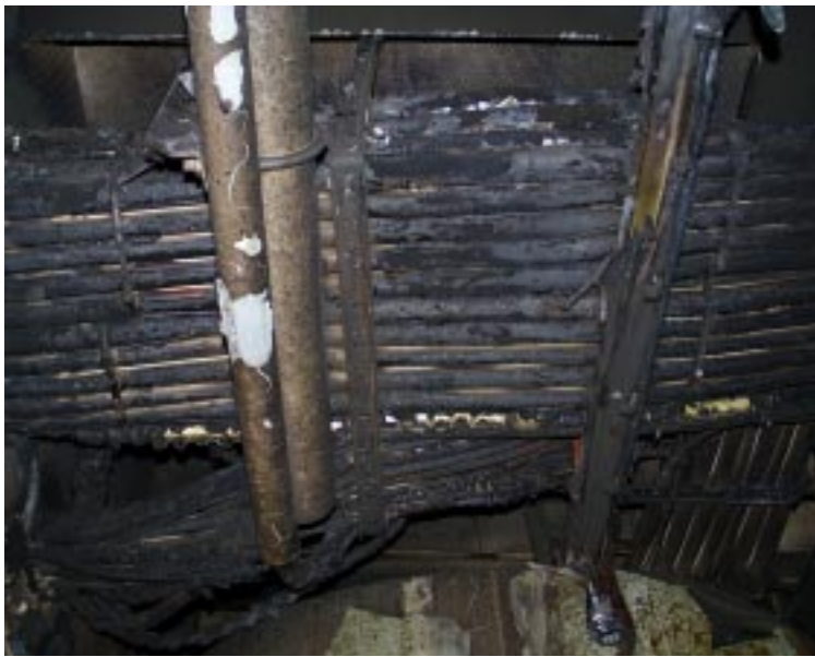
FIGURE 4 Fire damage to deckhead cables and fittings
