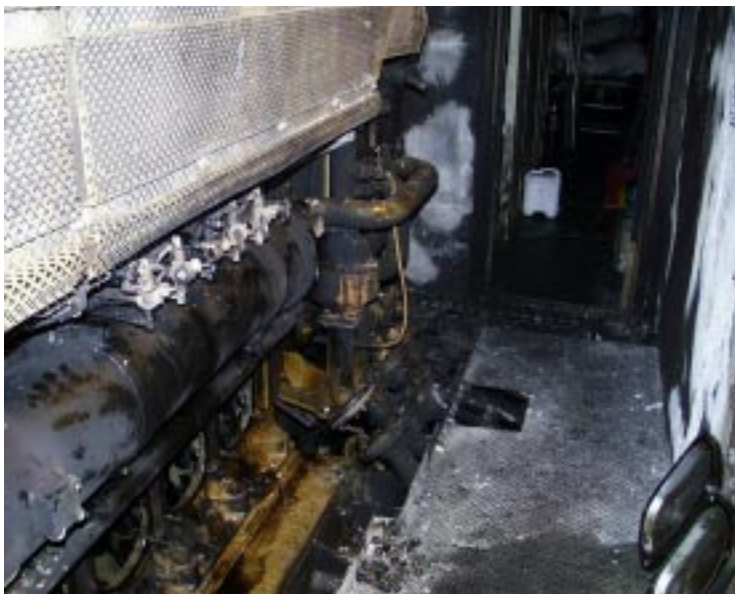
FIGURE 2 Port aft corner of generator space – bilge fire occurred here
