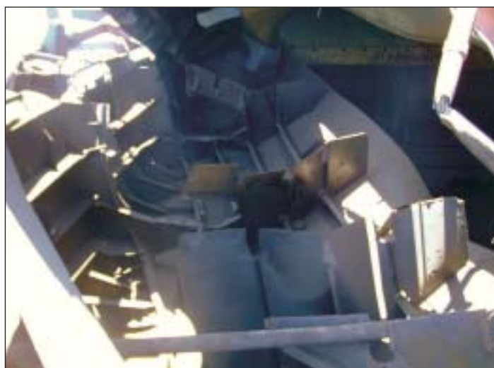
FIGURE 7: Interior of port topside ballast tank after the explosion
